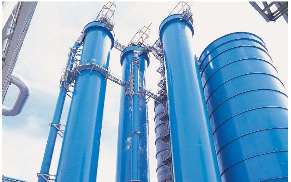
Four-stage ECF bleaching fiberline. Photo by Tom Grow, courtesy of Andritz AG.
